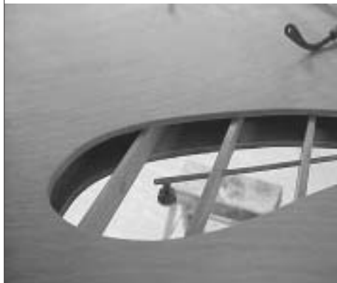
Throughout the house, there are cut-outs that allow viewers to see the fire sprinkler system.
