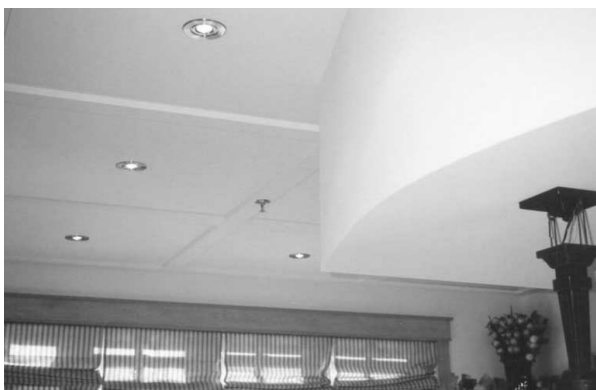
Visitors saw how inconspicuous sprinklers protect a house.
