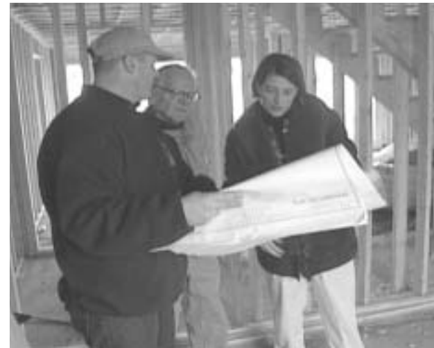
Katherine McGreen and her father, Laurence Ford, review the plans for her sprinkler system with David Walencewicz, P&J Sprinkler Co.
